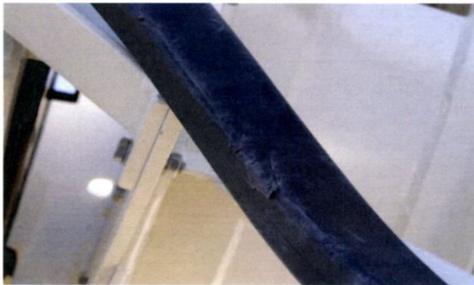
Figure 5 shows minor damage to the waveguide
